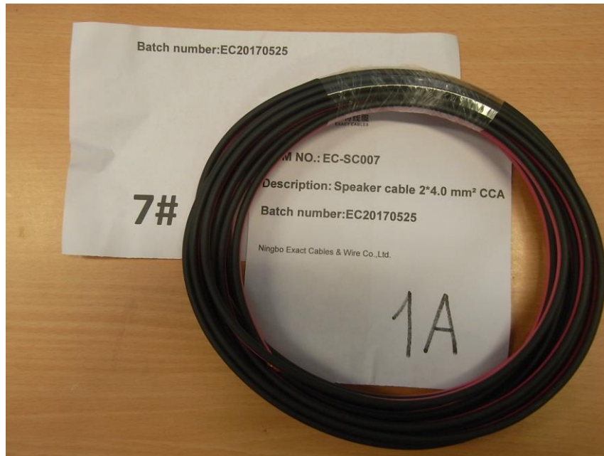
Cable/Cavo: SPEAKER CABLE 2x4,0 mm 2 CCA Marcatura/Marking: Non presente / Not present
